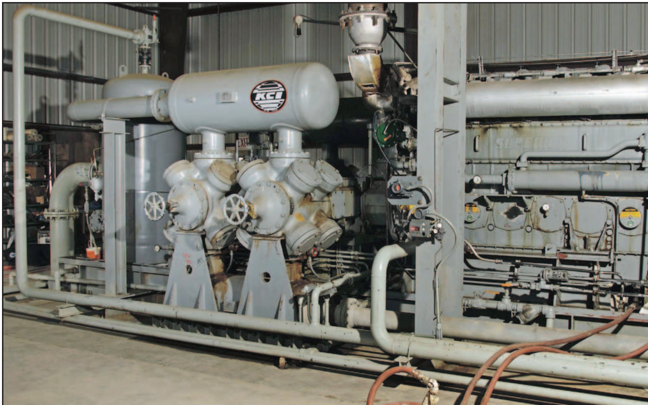
■ One of two Cooper/Superior Model 2406G natural gas-fueled engines rated at 1200 bhp (895 kW) at 1200 rpm at EnCana's Brighton compressor station. Each engine powers a Cooper Model 425CC natural gas compressor.
